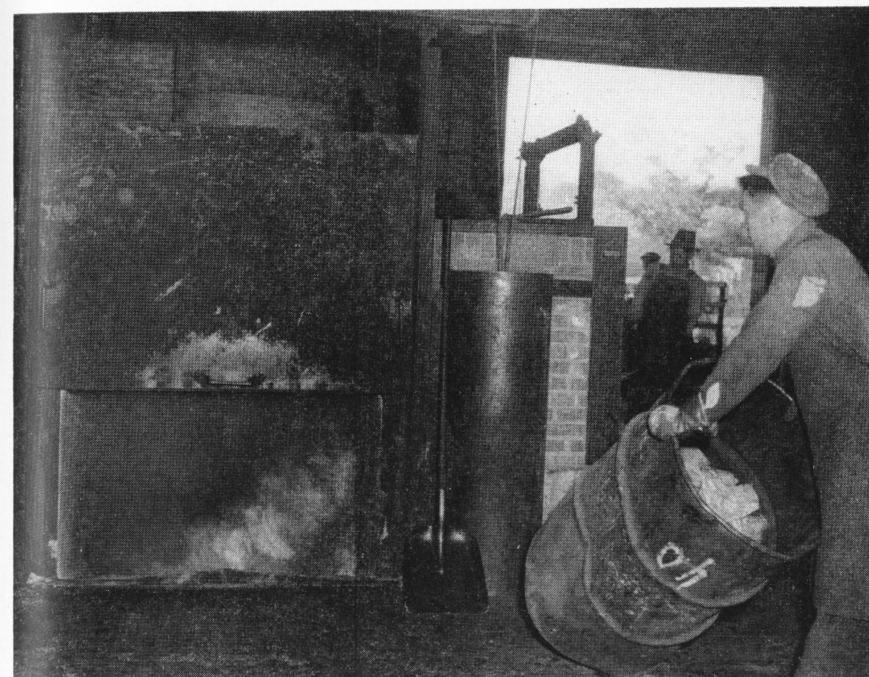
All combustible material is burned in this Morse-Boulger destructor furnace in Building 25. The ashes are shipped out to the refineries. On the job we see John Kuzio, C. Capozzi and Angelo Cantino.
