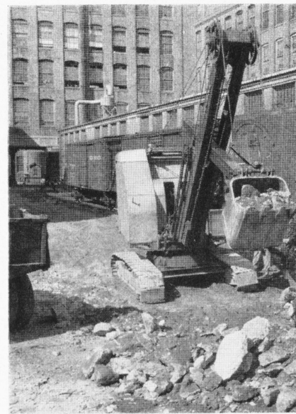
Power shovel and bulldozer team together on the job of tearing up Scovill's old streets. Solid cement on a strong base will replace the old roads.
